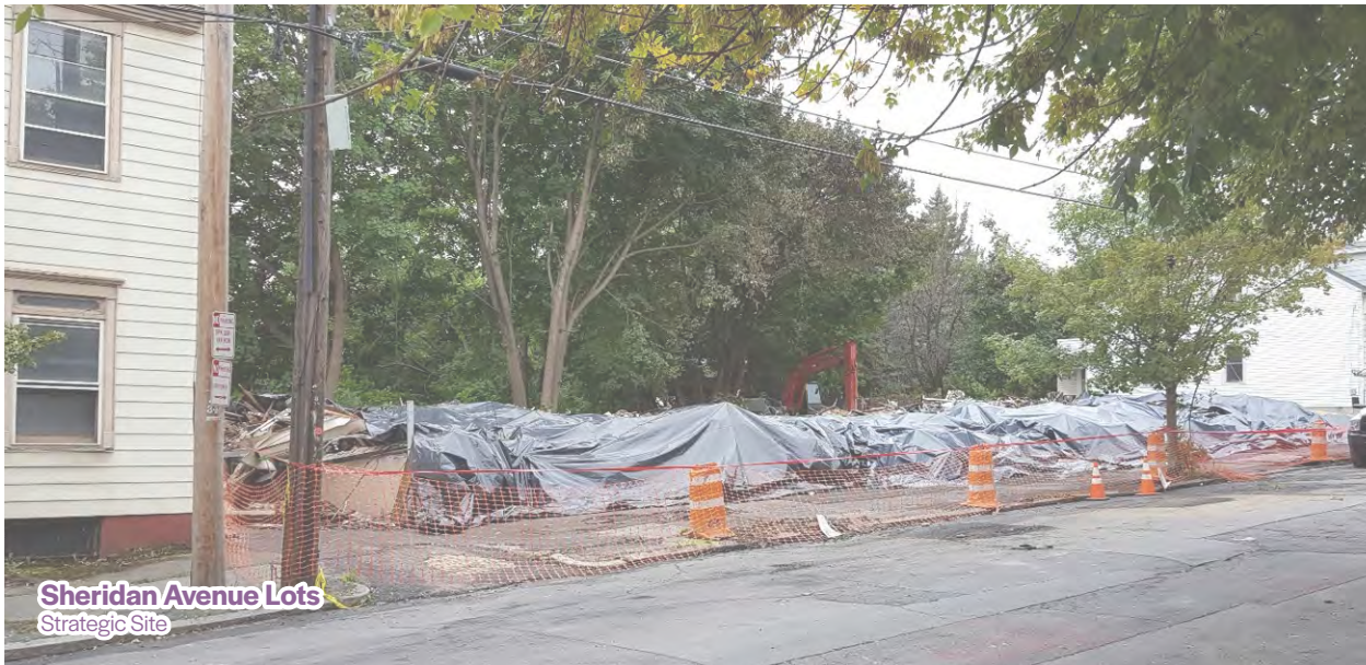
existing site after fire damage
